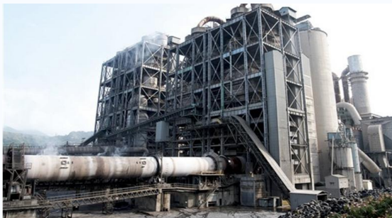
Cement: AI Heat Control for Preheater and Kil
